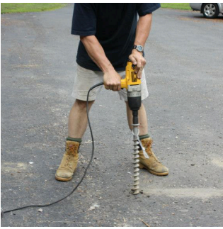
Pre drill pilot hole with impact wrench (this determines holding power). Earth Anchor can then be installed.
